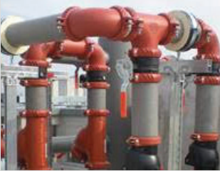
Water Delivery Systems
