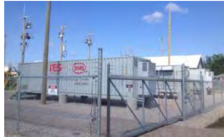
Canada RES 4MW/2MWh
