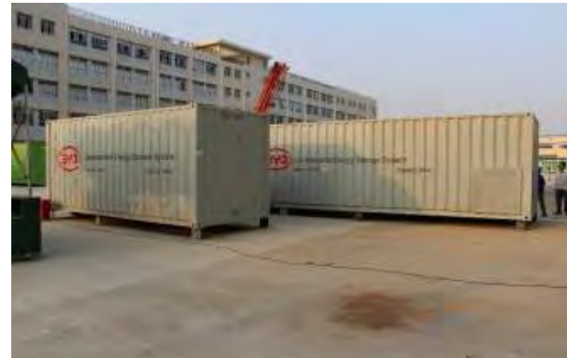
South Africa Eskom 200kW/1.2MWh
