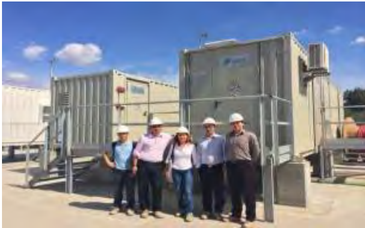
Italy Terna 2MW/2MWh
