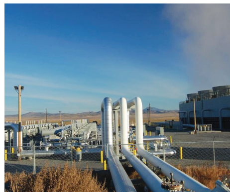
Thermo Hot Springs 14 MW
