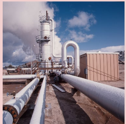
Blundell Geothermal Plant near Milford, Utah
