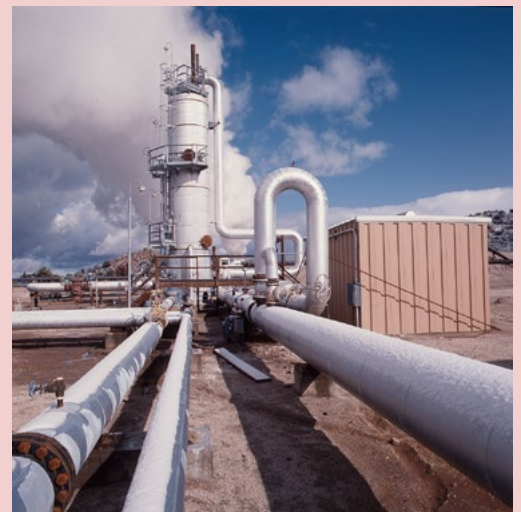
Blundell Geothermal Plant near Milford, Utah
