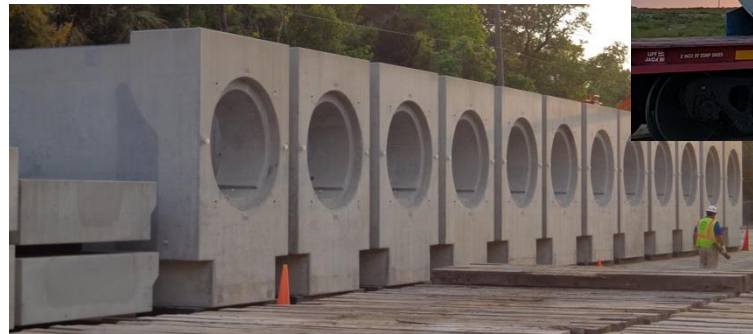
Horizontal storage modules for used nuclear fuel. Photo Credit: Crystal River Site.
